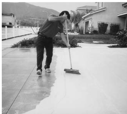
Continue spreading the material ahead of the person brooming using the metal squeegee.
