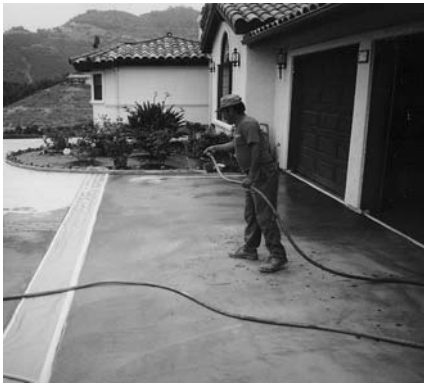
1. Make sure surrounding areas are taped off and fog the surface with water where you wish to begin spreading the material.
