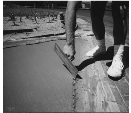
4. Scrape out any material that got in the joints using a trowel or scraper before it dries too hard. Apply Concrete Colorcoat using a paint roller.
