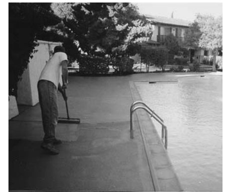
5. After blowing off the surface, apply two coats of Concrete Colorcoat w/a paint roller.
