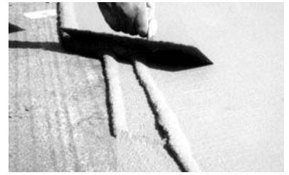
Patch holes or areas needing repair
