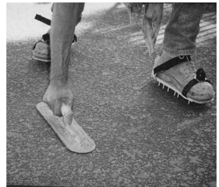
3. While wearing spiked shoes knock the spray texture down flat before it dries using a trowel.
