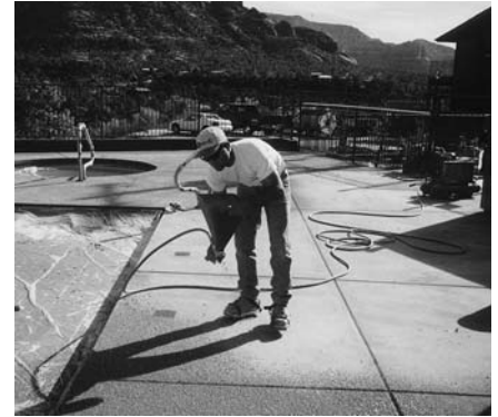
Spray the Trowel Knockdown Mix over the surface using hopper gun spray unit.
