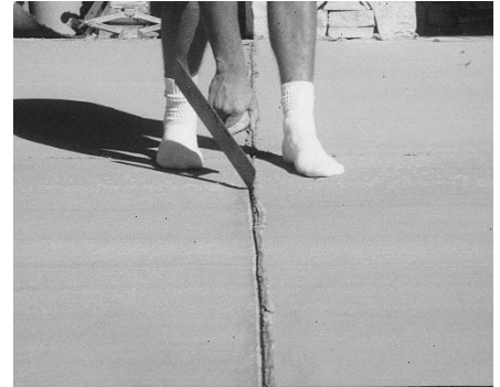
4. Scrape out any material that got in the joints using a trowel or scraper before it dries too hard.
