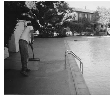
5. After scraping and blowing off the surface, apply two coats of Colorcoat 100 w/a paint roller.
